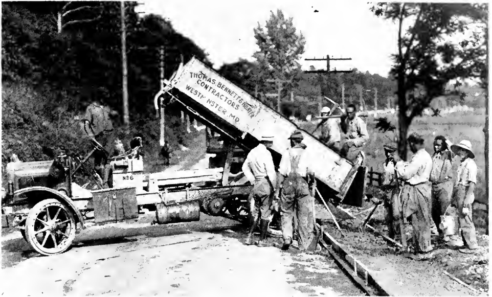
Concrete shoulders not only widened the roadway but allowed for strengthening the surface. The space between the raised shoulder and the center or crown of the road will be filled with road material.
